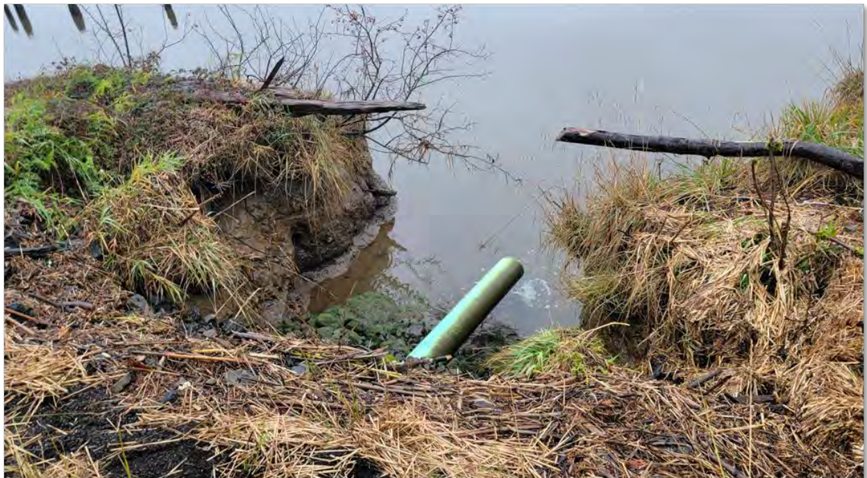
Figure 12. Severely eroded shoreline around assumed stormwater outfall pipe.
